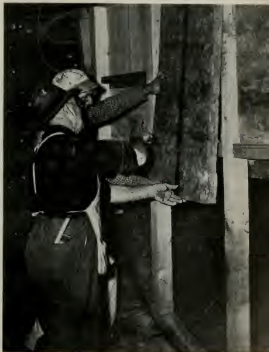
Cutting the Fiberglas insulation to fit the space between the studs of the bulkhead separating the hold and the combined galley and fore-castle.
